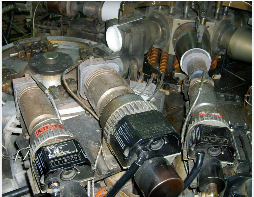
Production line with two LE 10 000 S and one LE 5000.
