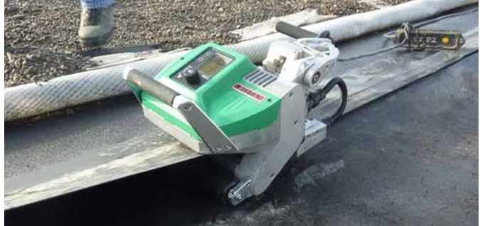
The GEOSTAR welds nearly 240 m without difficulty in a single pass during a field test (South Africa)..
