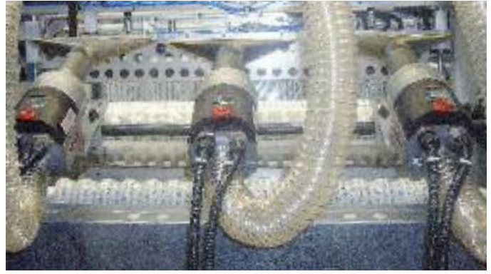
Three LHS 60S air heaters with wide slot nozzles in a wrapping line.
